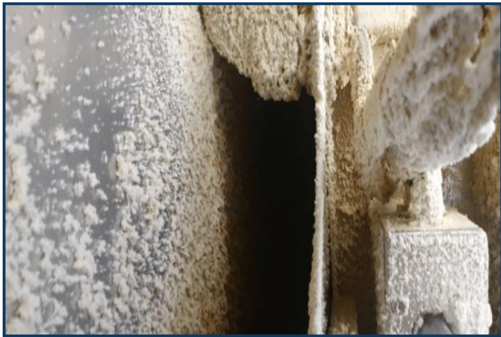
Photo from the ventilation system
