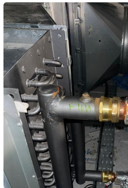
Supply Air Intake Coil
