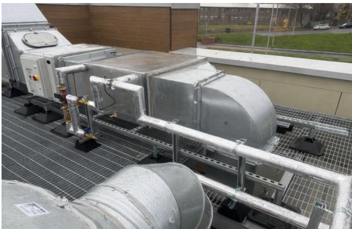
Rooftop Exhaust with Lepido installed in existing duct prior to the filtration & scrubber
