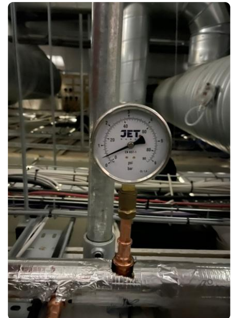
Piping with Measurement
