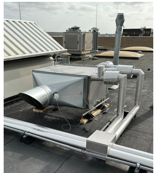
Rooftop Exhaust with Lepido directly venting to atmosphere
